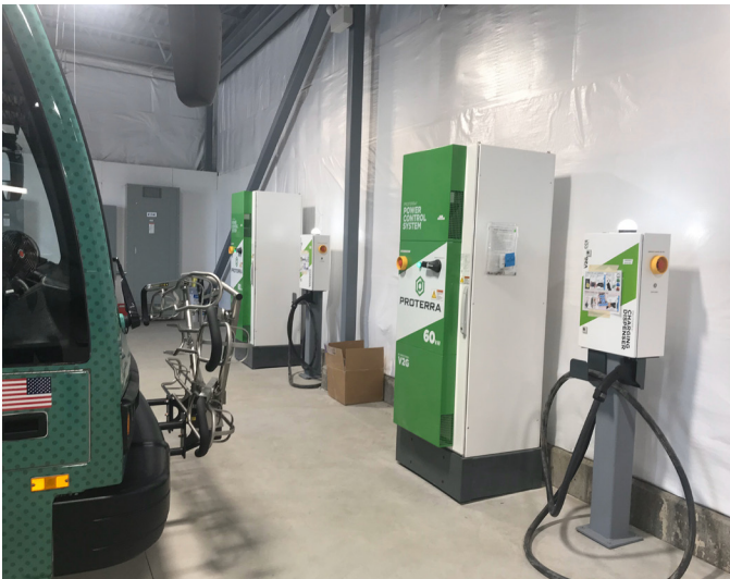
Electric bus charging station inside the Free Ride bus barn
